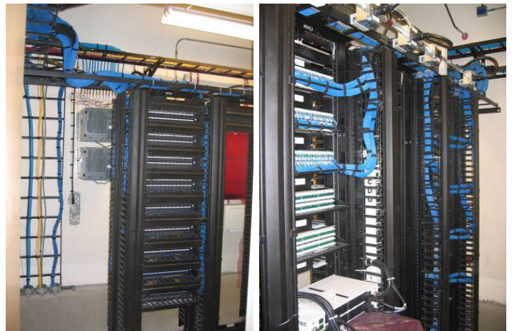
Figure 5 – Typical TR Racks, Cabling, and Equipment
